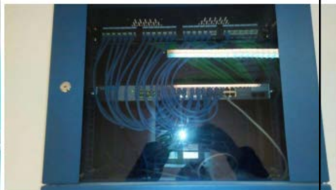
SG0046 RACK ZONA A AULA 2-10
